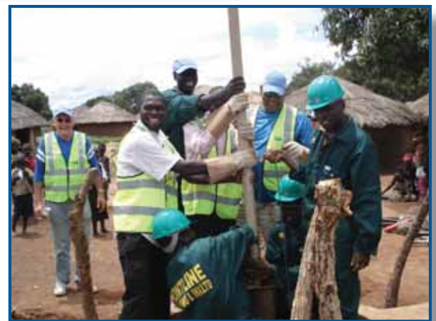
Above, Frederick (tallest) and FRONTLINE crew, Rotarians, Rotaractors installing the PVC Pipes into the aquifer ready for compressor development.
